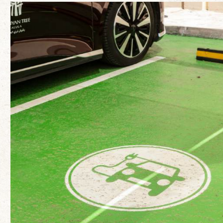
Installation of charging stations to support a fleet of electric vehicles - RCU Campus
