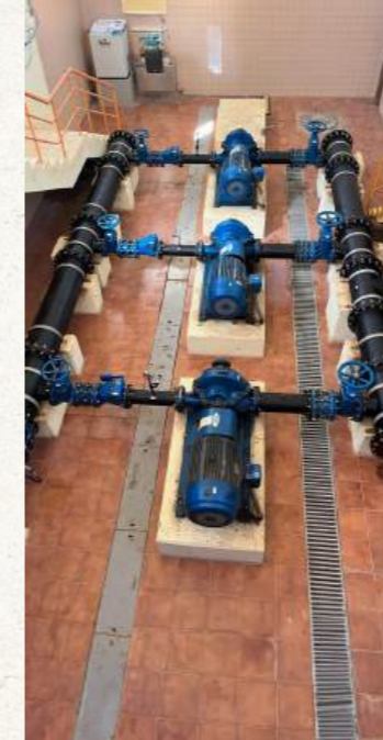
Water treatment facilities - Ashar Valley
