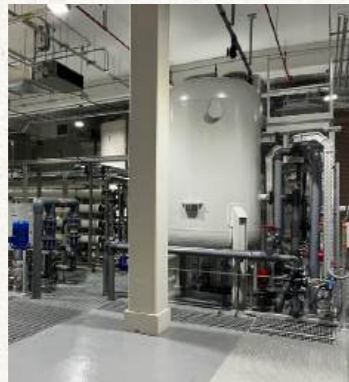
Water treatment facilities - Ashar Valley
